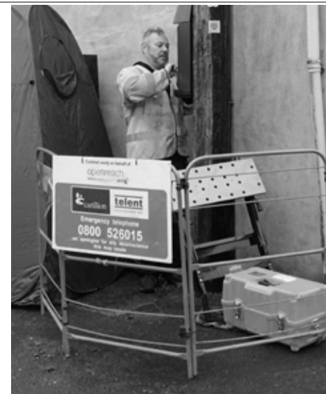
As we went to press, engineers were in Marshwood working on installing superfast connections.
